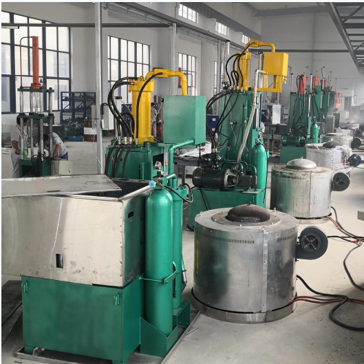
500Kg Al holding furnace *14 sets
